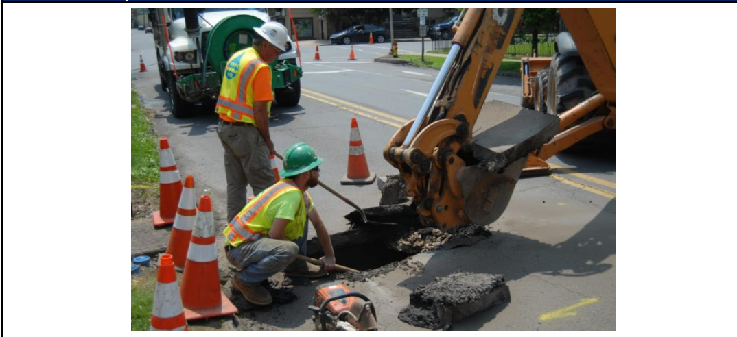
Figure 4.3.10-2 Large Sinkhole caused by sewer break in the City of Williamsport (Danneker, June 1, 2019).
