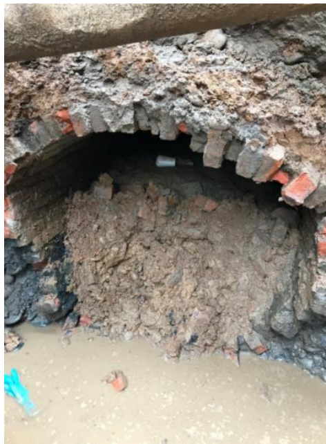
Figure 4.3.10-3 Large Sinkhole caused by sewer break in the City of Williamsport (Danneker, June 14, 2019).
