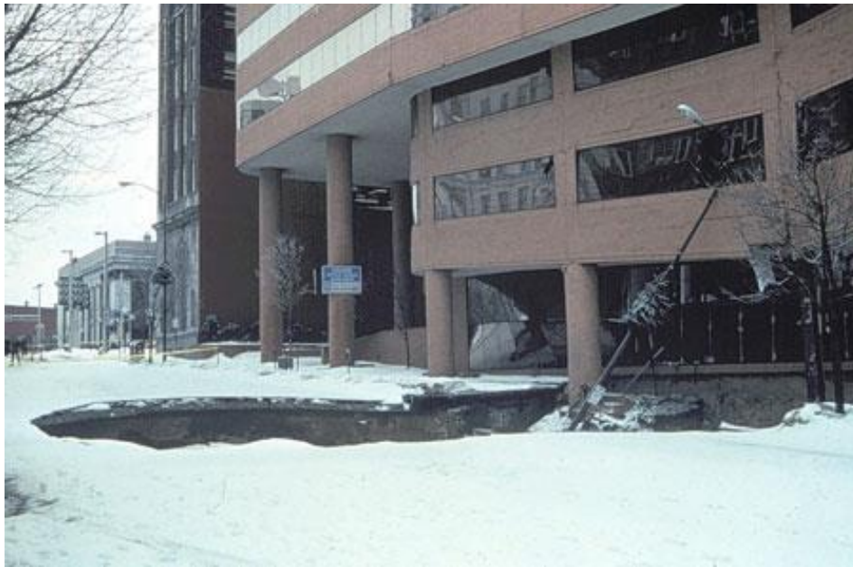
Figure 4.3.6-2 Sinkhole at Corporate Plaza Building in Allentown, Lehigh County, PA in February 1994 (Photography by William E. Kochanov – DCNR, 2009)
