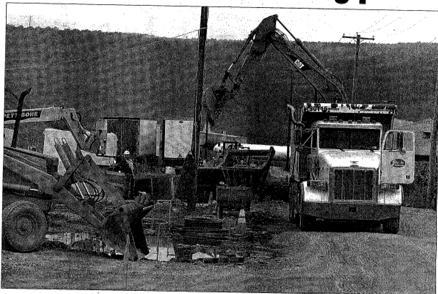
Construction continues on sewer lines for the Tiadaghton Valley Municipal Authority's treatment plant in Nippenose Valley. Another view appears on Page A-1. KAREN VIBERT-KENNEDY/Sun-Gazette
