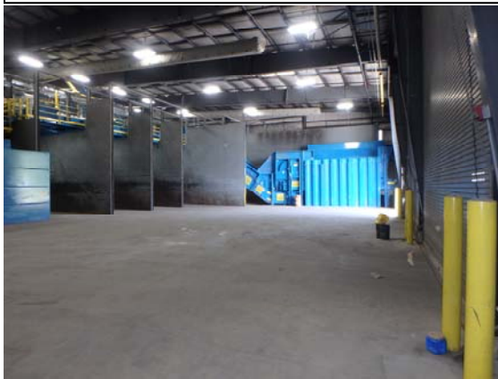
Tipping floor with metering bin
