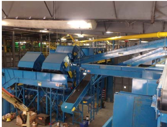
Over-view of the main sorting conveyor system
