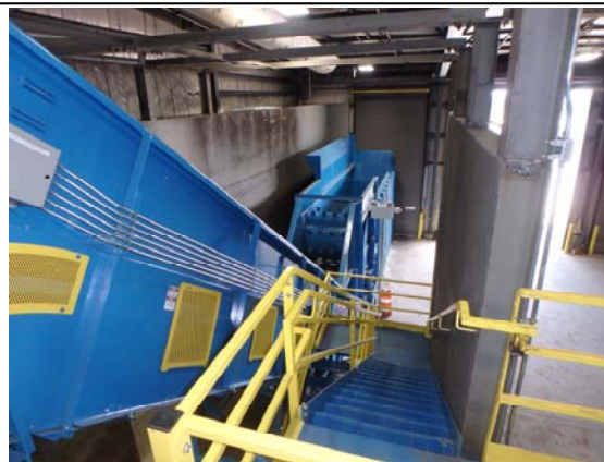
Conveyor from the metering bin to the pre-sort line.
